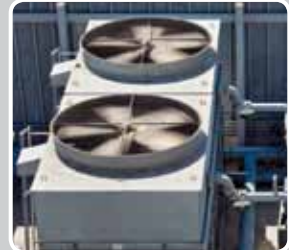
- Rooftop Cooling Units - Emergency Generators
